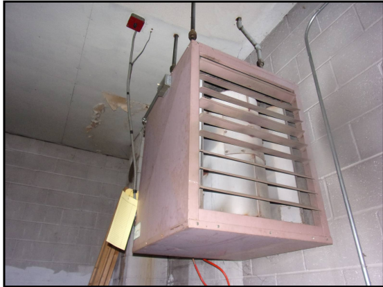
73: Space heater in Fire House
