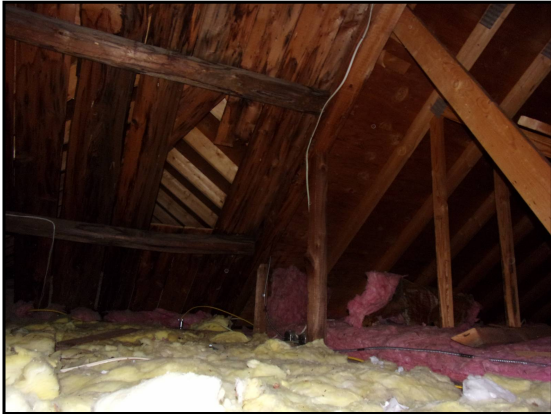
61: Attic area in Town Hall located under the connecting roof to Admin Offices
