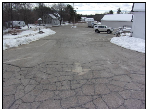
24: Distressed pavement / alligator cracking near Fire House
