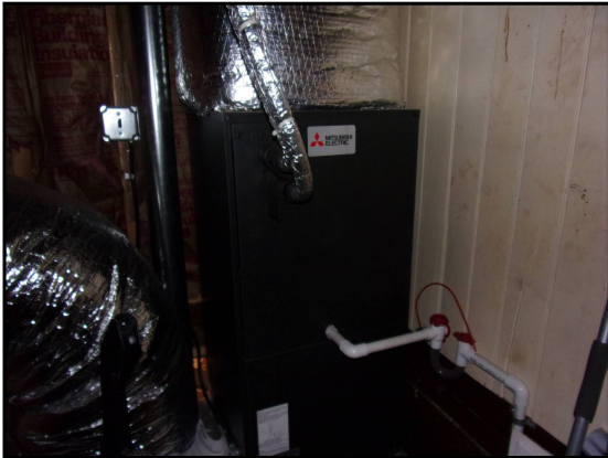
51: Interior HVAC in Town Hall
