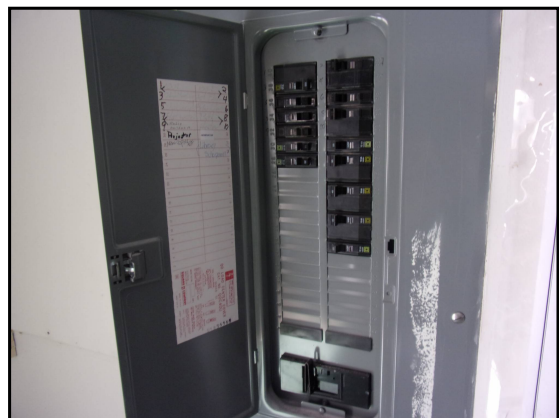
78: Typical breaker panel
