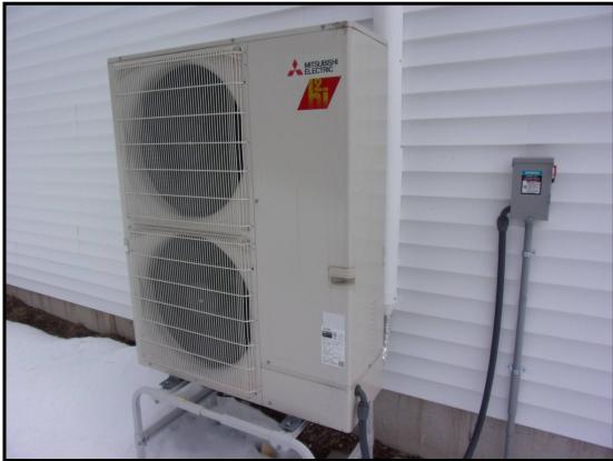
9: Exterior mini-split condenser unit
