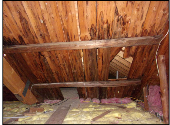
62: Opening in Town Hall roof to attic of connecting hallway
