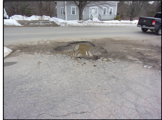
26: Large pothole near Fire House
