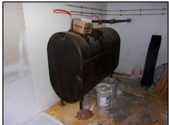
72: Fuel oil tank in Fire House
