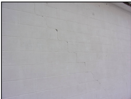
17: Step-down cracking in exterior CMU of Fire House
