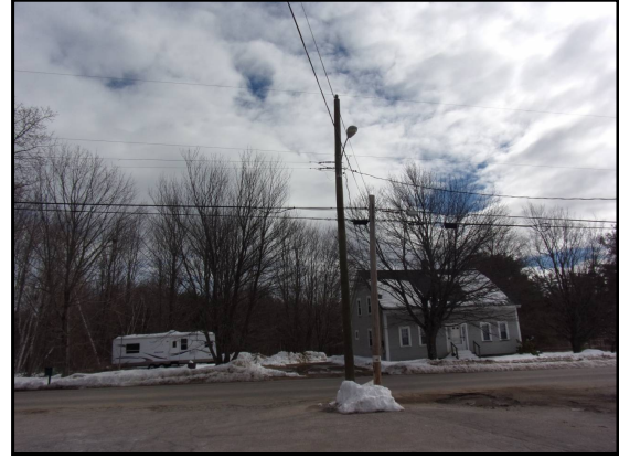
32: Electrical service and pole-mounted lighting
