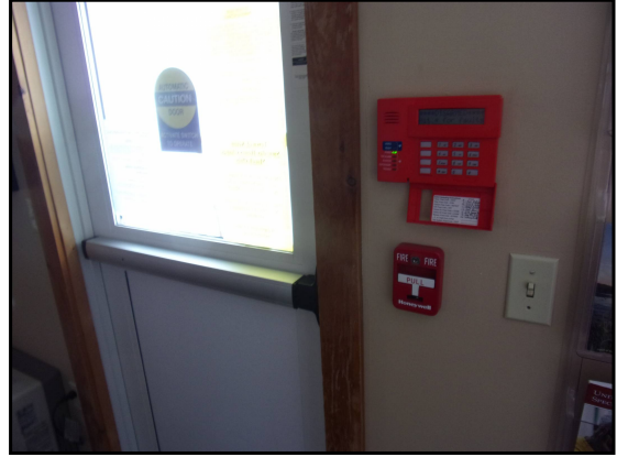
44: Exterior door with alarm stations
