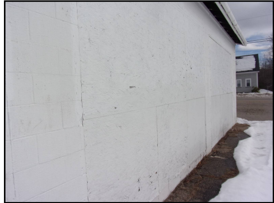
20: Boarded up truck bay
